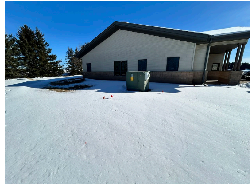
The existing transformer on the west side of the existing building.
