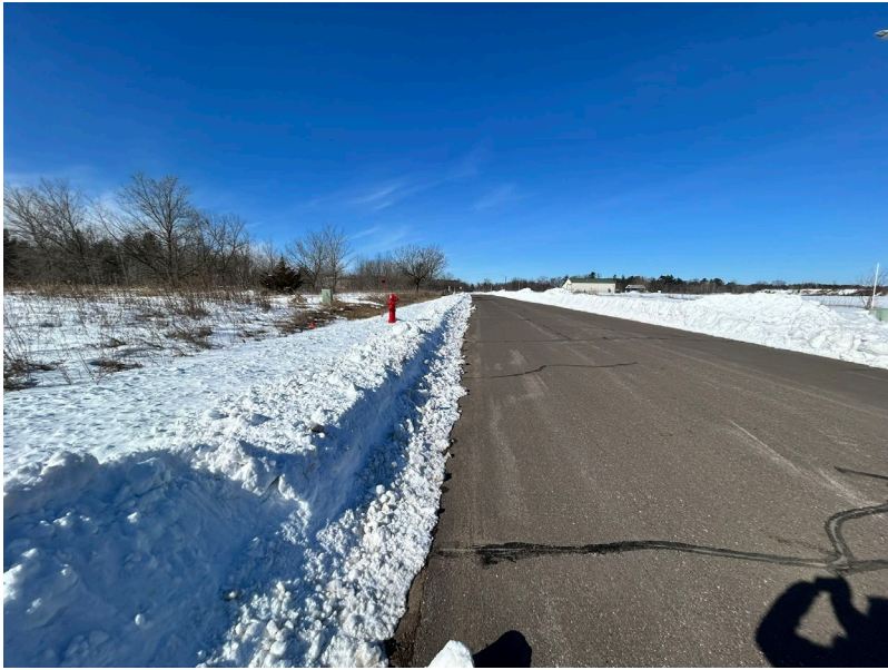
Fire-hydrant across Guy Ave, near the southwest corner of the west driveway.
